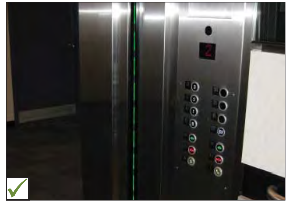
Elevator sensor door and floor registration buttons.
