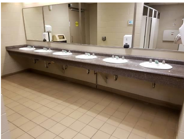
View showing the condition of the sinks and countertop in the washrooms.
