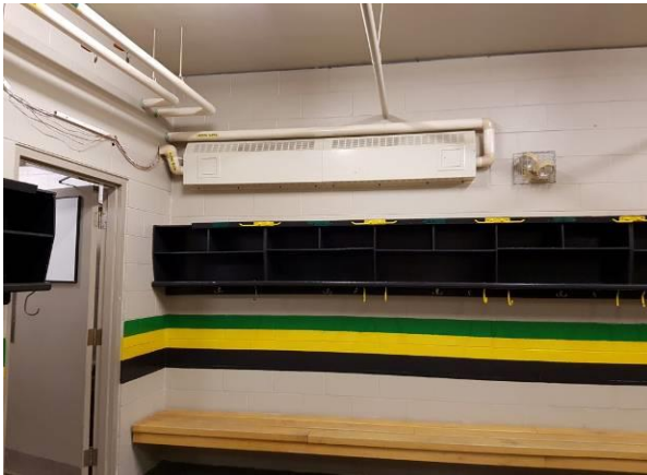
View showing the condition of the wall mounted heaters in the change rooms.
