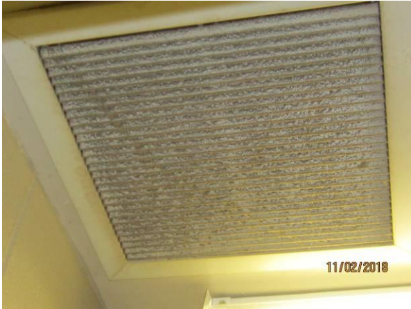
View showing the condition of the ceiling exhaust vent in the washrooms – change rooms.
