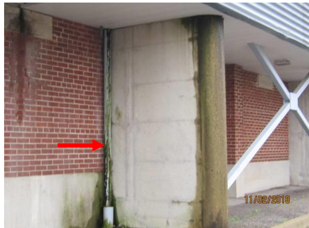
View showing the condition of the broken downspout at the north elevation.
