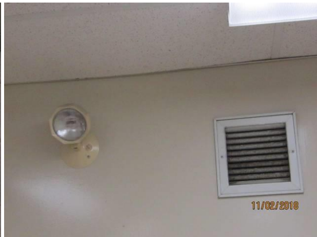
View showing the condition of the emergency light in the building.
