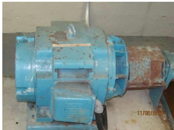
View showing signs of corrosion on the pumps.
