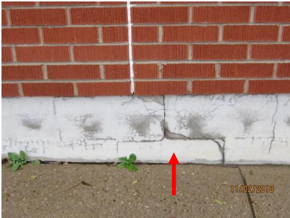
View showing cracks in foundation walls above grade.
