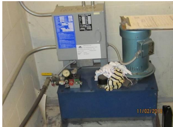
View showing the condition of the elevator machine in the ground floor.
