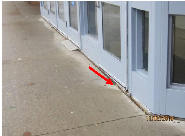
View showing missing sealant between concrete slab and building wall at the east elevation.
