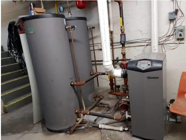
View showing the condition of the the boiler and water tanks in the sprinkler room.
