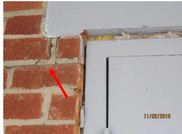
View showing cracked mortar joints in the brick veneer near exterior door at the south elevation.
