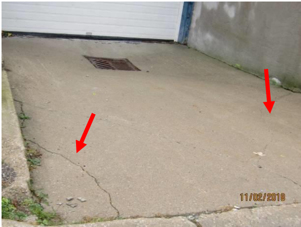
View showing cracked concrete slab in front of overhead door at the west elevation.
