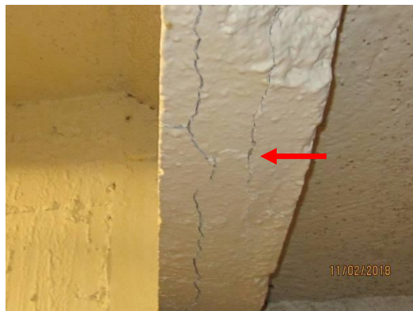
View showing cracks in the concrete beam in the ground level.
