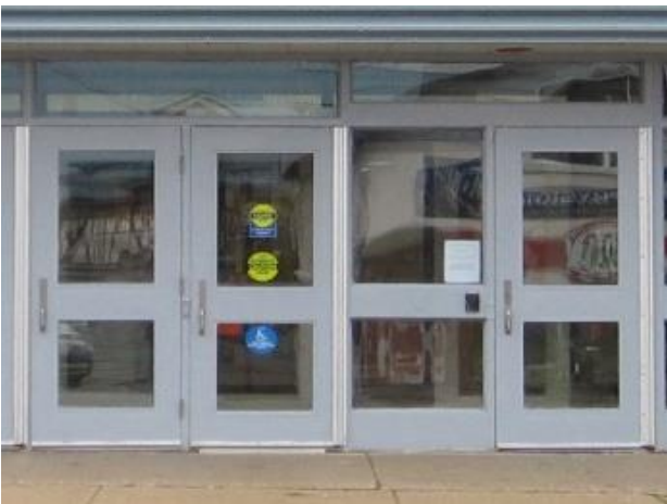
View showing the condition of the main entrance door.
