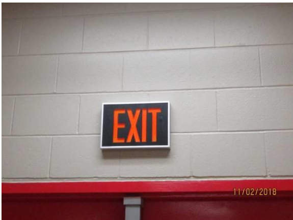
View showing the condition of the lighted exit fixtures in the building.
