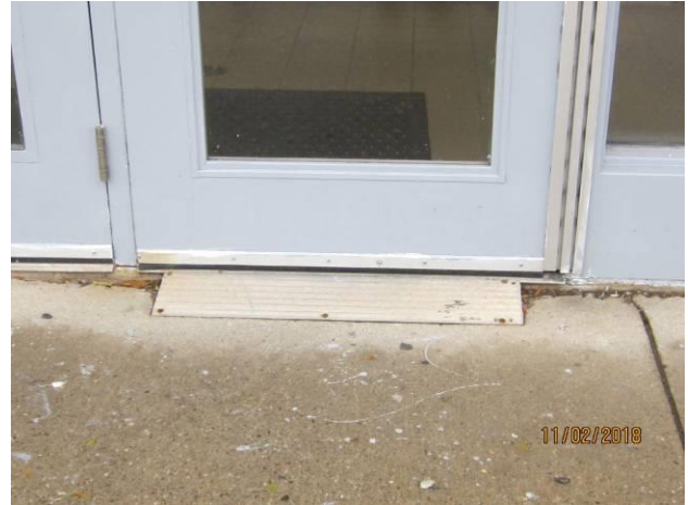
View showing a small ramp at the front entrance door (accessible door).
