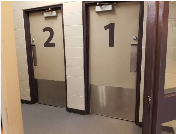
View showing the condition of the interior single metal doors for change rooms.
