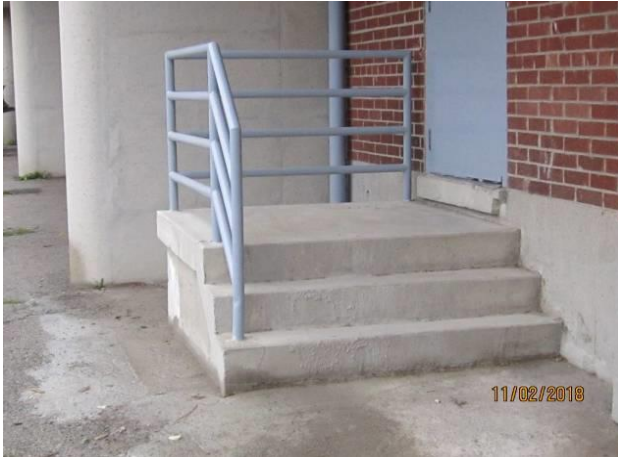
View showing the condition of concrete steps at the south elevation.
