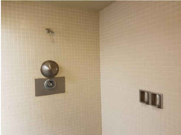
View showing the condition of plumbing fixtures in the shower area.
