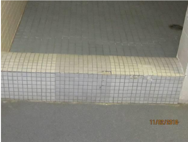
View showing the condition of the ceramic tiles in the shower area.
