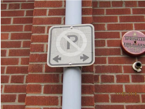
View showing the condition of faded parking sign.
