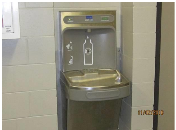
View showing the condition of the drinking fountain in the building.
