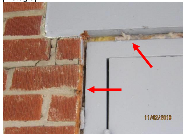
View showing missing sealant around door frame at the south elevation.
