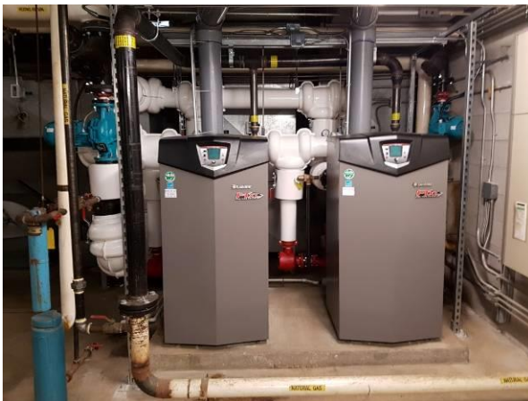
View showing the condition of the boilers in the penthouse.
