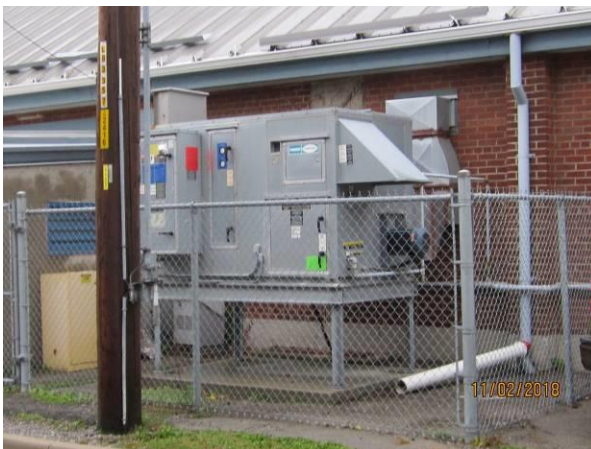
View showing the condition of the air-handling unit west side of the building.
