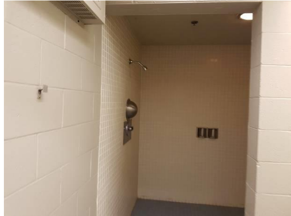
View showing the condition of the ceramic wall tiles in the shower area and painted block walls in the change rooms
