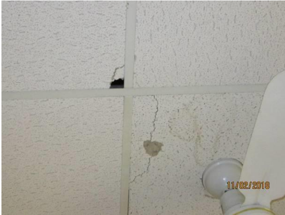
View showing a broken ceiling tile in the storage area.
