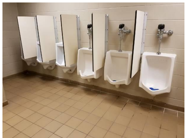
View showing the condition of the urinals in the washrooms.
