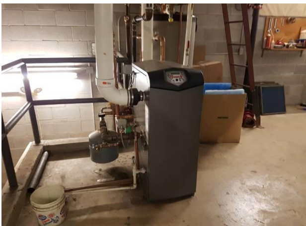
View showing the condition of the boiler in the penthouse.
