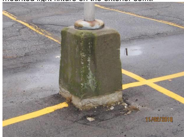
View showing damaged concrete base for pole-mounted exterior lighting.
