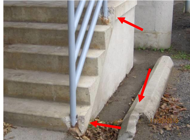
View showing chipped concrete at the connection of the handrail on the exterior stairs and broken wheel stops.
