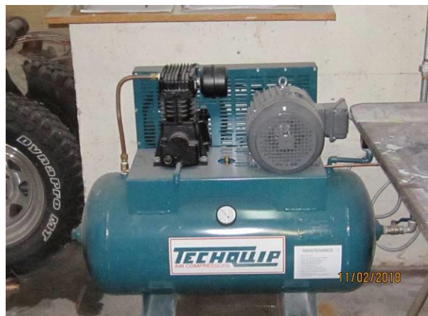
View showing the condition of the air compressor.
