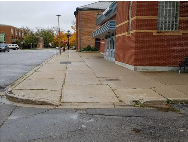
View showing the condition of the concrete slab in front of the building.
