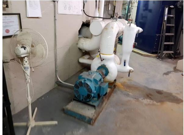
View showing the condition of the pipes and pumps in the refrigerator room.
