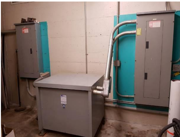
View showing the condition of the transformer and breaker panels in the main electrical room.
