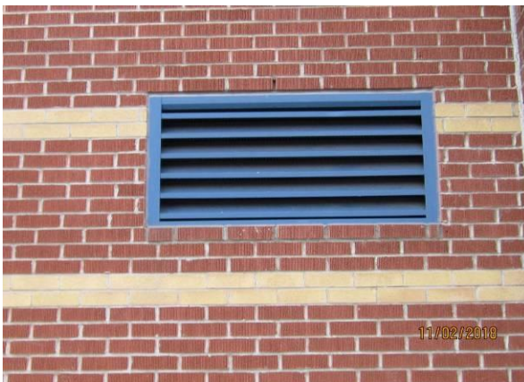
View showing the condition of the vent cover on the exterior walls.
