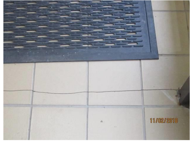
View showing cracked ceramic tiles in the vestibule area.
