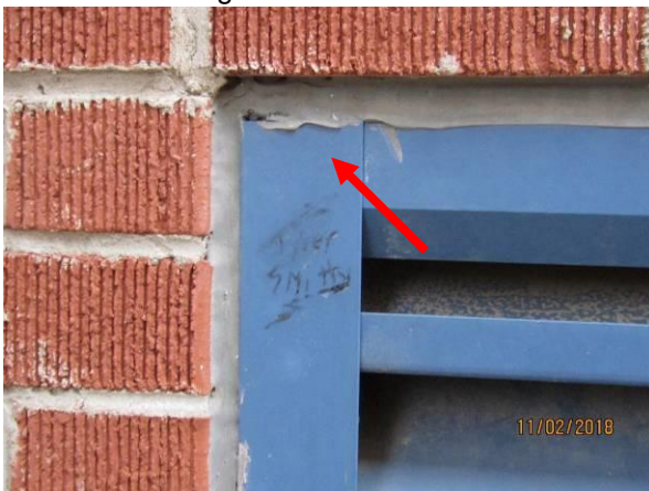
View showing damaged sealant around exterior louver.
