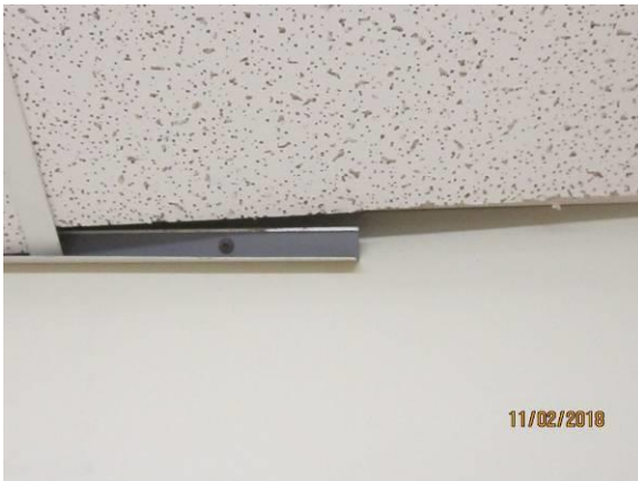
View showing broken tile frame in the third floor.
