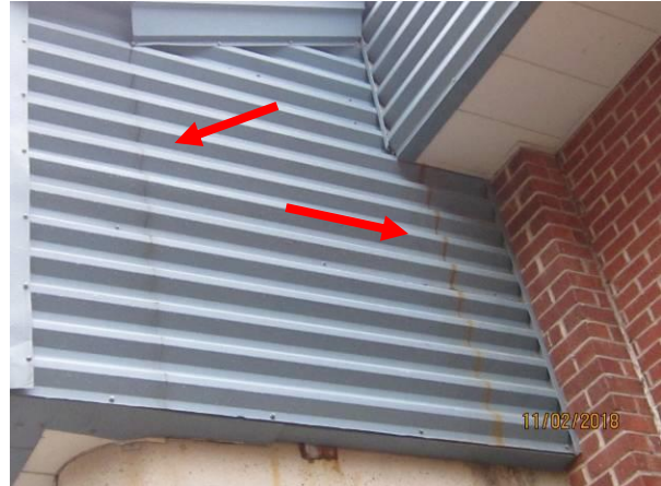
View showing rust stains on the metal cladding at the south elevation
