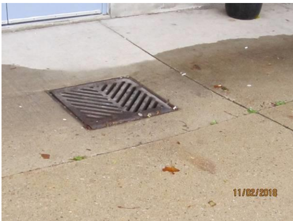
View showing the condition of the catch basin in front of the building.
