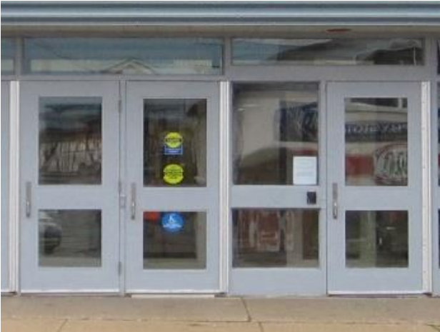
View showing the condition of the main entrance.
