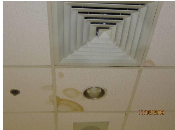
View showing typical stains on ceiling tiles.
