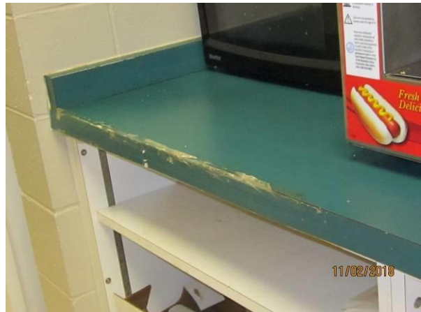
View showing damaged countertop in the Concession Room.
