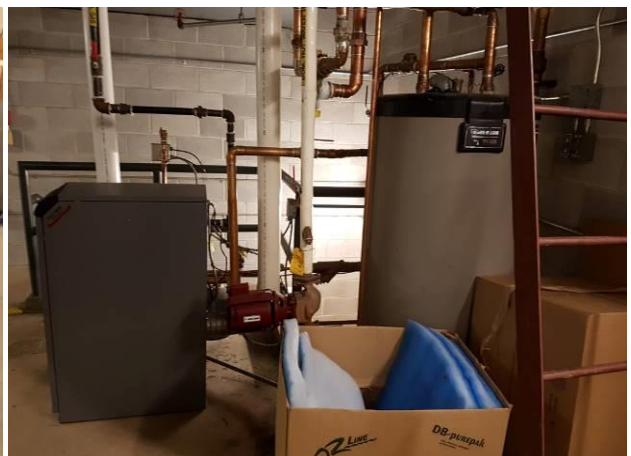
View showing the condition of the boiler and water tank in the penthouse.
