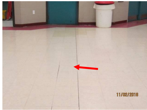
View showing gaps/separation in vinyl flooring.
