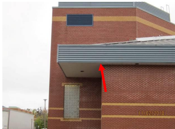
View showing the condition of the metal soffit and fascia.
