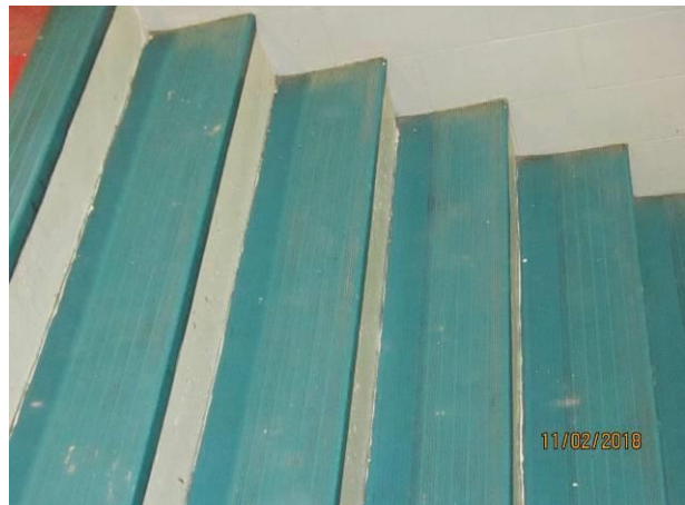
View showing the condition of the stair's cover at the east side of the building.
