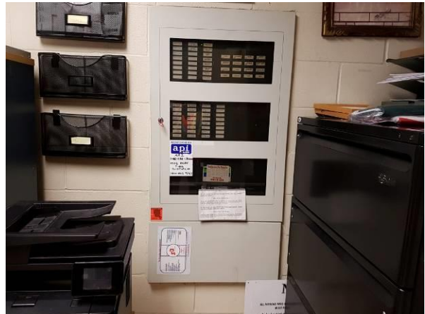
View showing the condition of the fire alarm panel in main/front office.
