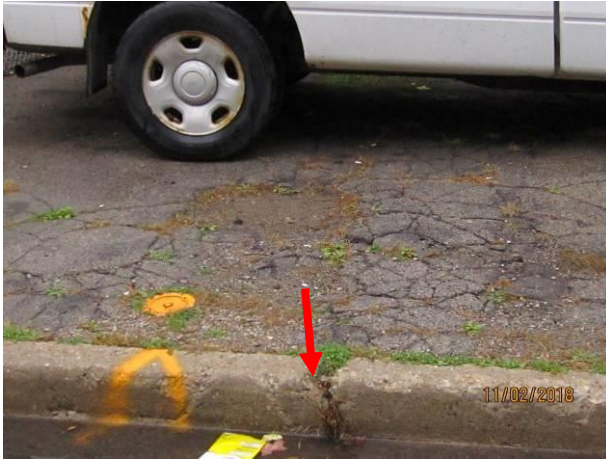
View showing broken curbs and damaged asphalt pavement at the west side of the building.
