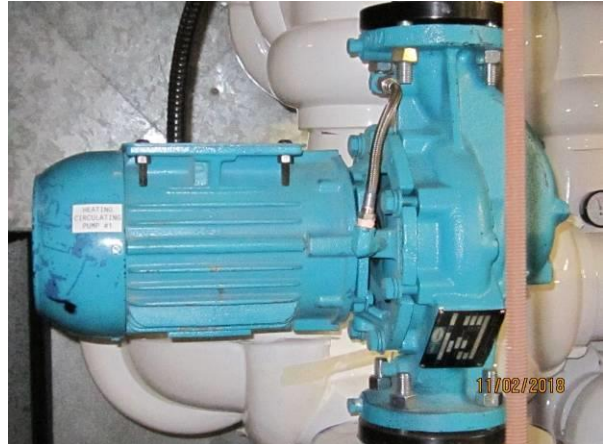
View showing the condition of the pumps.
