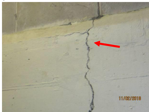
View showing vertical cracks in foundation walls in the service area.
