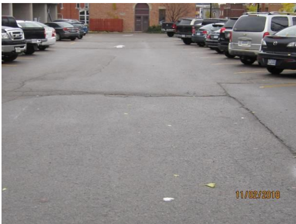
View showing the condition of the south parking lot.
