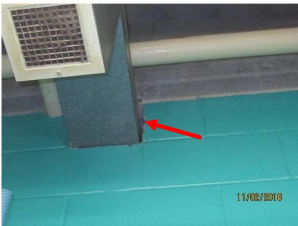
View showing missing smoke and firestopping around duct in concrete block walls
