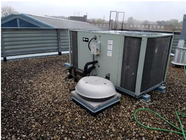
View showing the condition of the HVAC unit on the flat roof.
