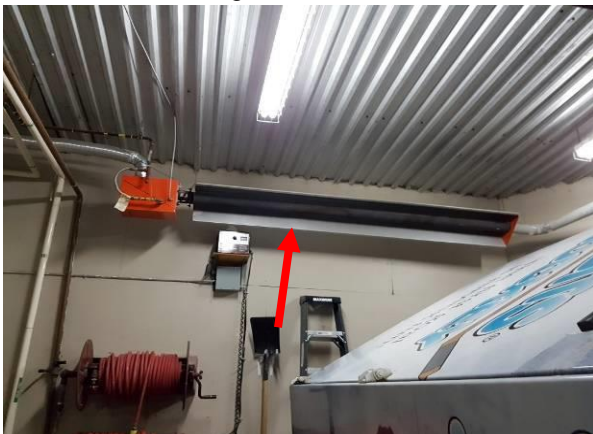
View showing the condition of the ceiling mounted heater in the zamboni room.
