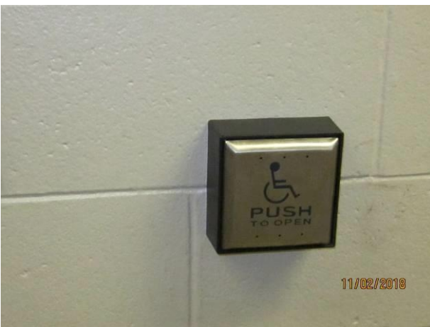
View showing the automatic door opener inside the building.
