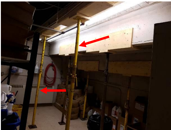
View showing metal posts supporting cracked concrete beams.
