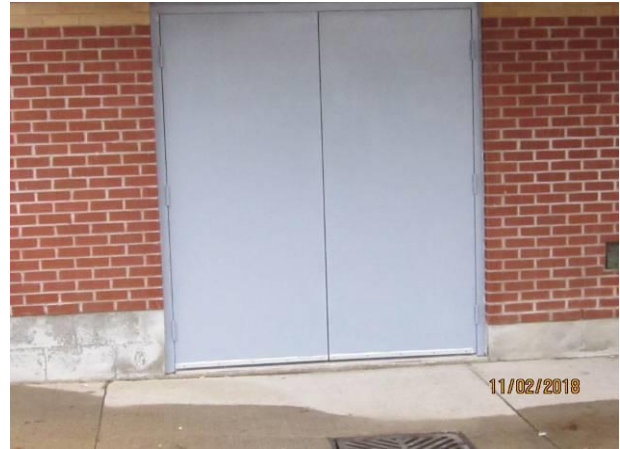
View showing the condition of the metal service double door.
