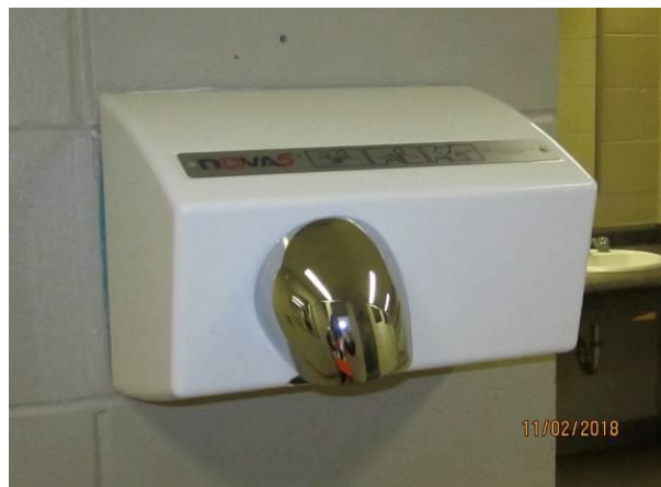
View showing the condition of the hand dryer in the washrooms.
