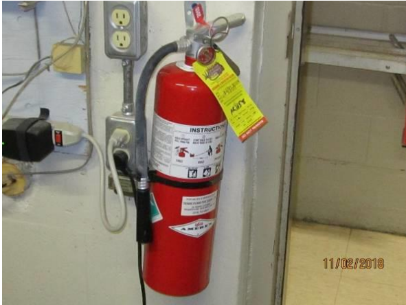
View showing typical condition of the fire extinguishers.
