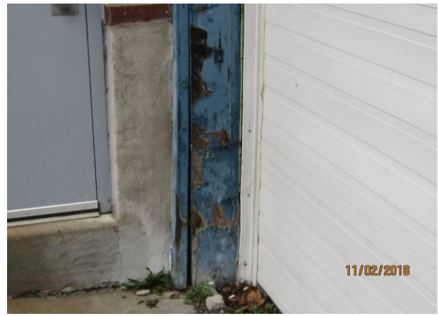
View showing rotten wood frame for overhead door.
