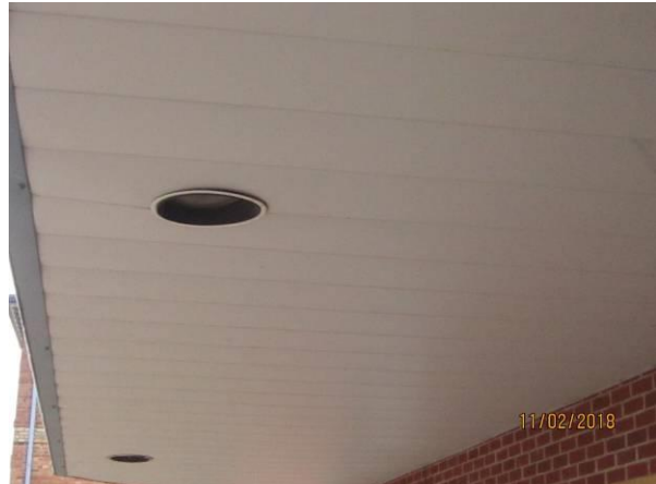
View showing the condition of the front canopy's soffit.
