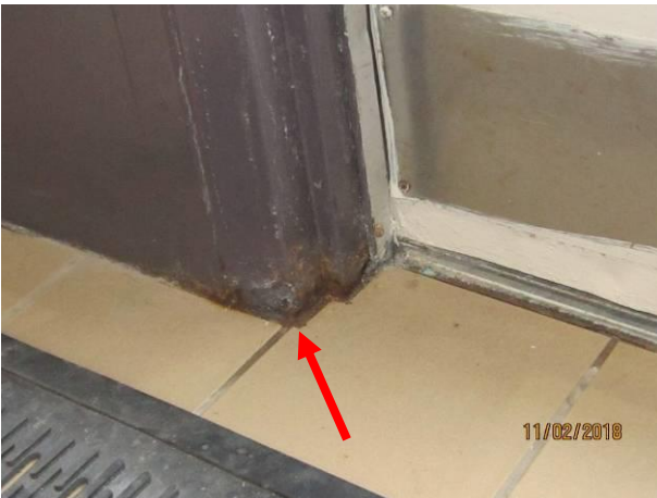
View showing corroded metal frame at the entrance door.
