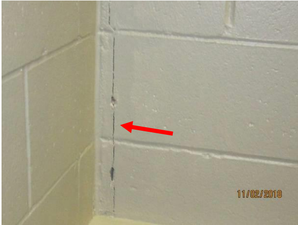
View showing vertical crack in concrete block walls.
