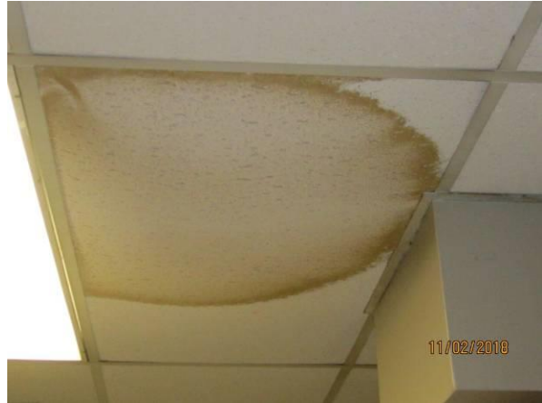
View showing stains on ceiling tiles in the women's washroom.
