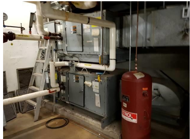
View showing the condition of two air handling units in the penthouse.
