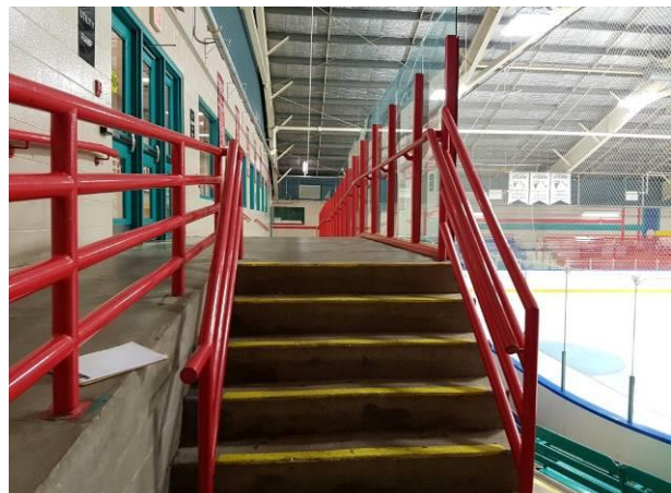
View showing the condition of the stairs, metal handrails and the concrete ramp in the Arena area.
