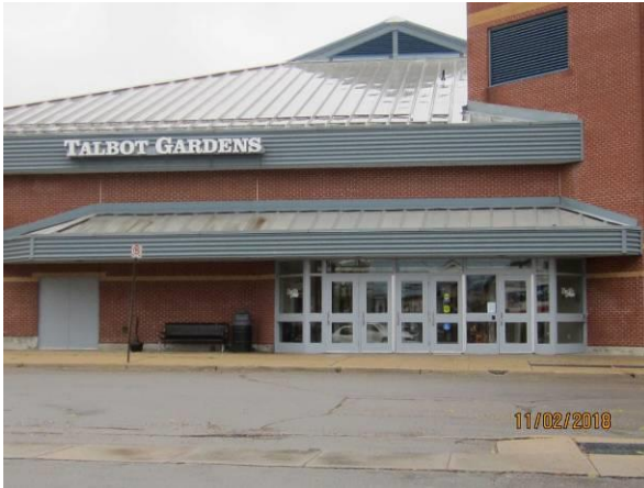
View showing the condition of the front canopy above the main entrance.
