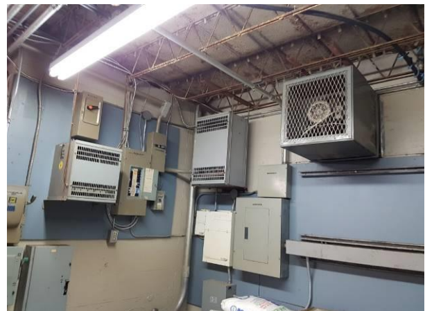
View showing the condition of the wall exhaust fan in the service room.
