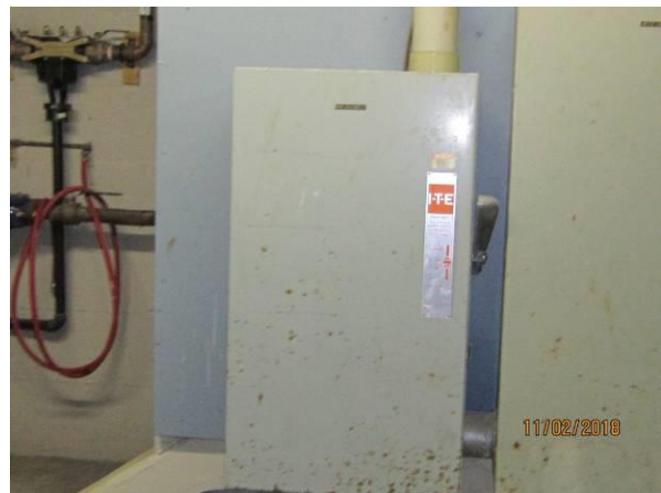
View showing the condition of the main disconnect.
