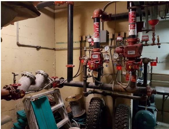
View showing the fire sprinkler system and valves.
