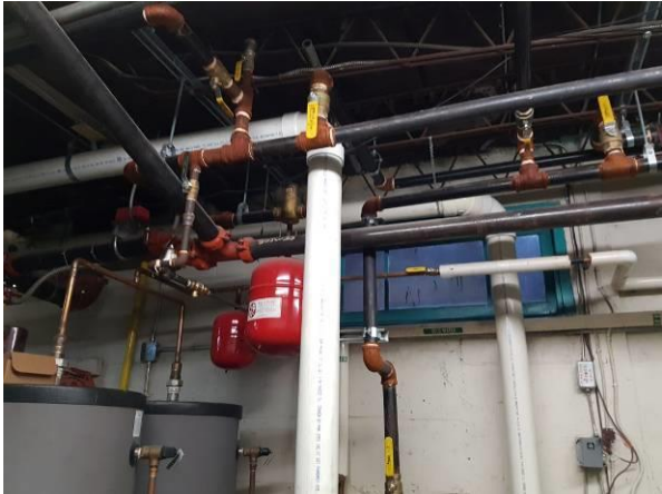
View showing the condition of the pipes and expansion tanks in the sprinkler room.
