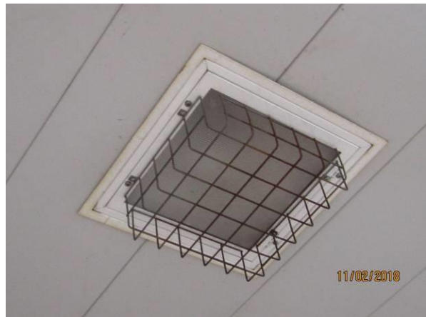
View showing the condition of the ceiling mounted light fixture on the exterior soffit.
