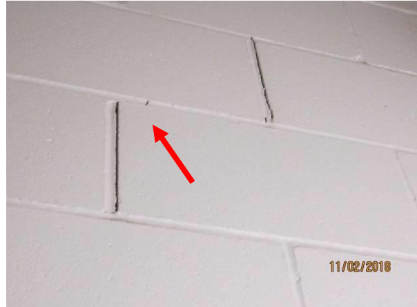
View showing step crack in concrete block walls at stair well leading to music room – third floor.
