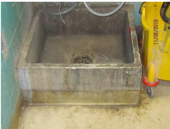
View showing the condition of floor sink in the janitor room.
