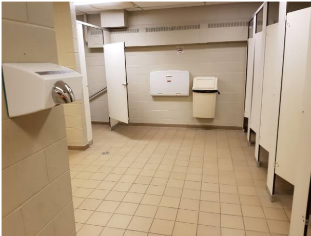
View showing the condition of the ceramic tiles in the washrooms.
