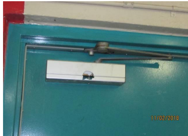
View showing the condition of the auto closer for exit and service doors.
