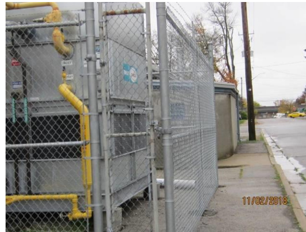
View showing the condition of the chain-link enclosure at the rear elevation around mechanical units.
