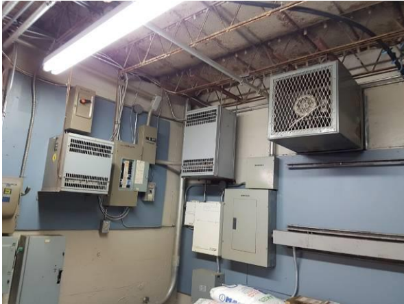
View showing the condition of the transformers and electrical panels in the refrigerator room
