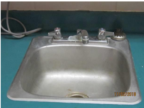
View showing the condition of the stainless steel sinks in service rooms.
