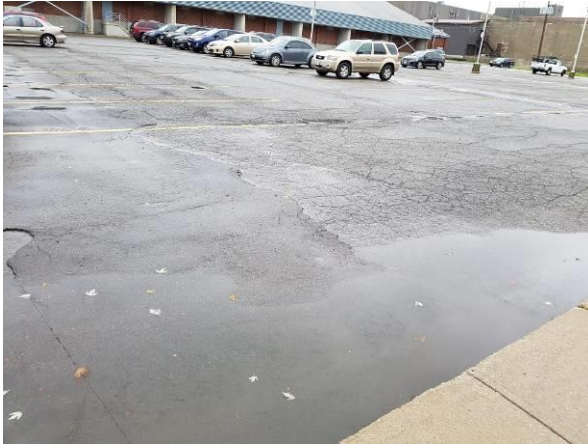
View showing the overall condition of the asphalt pavement with standing water.
