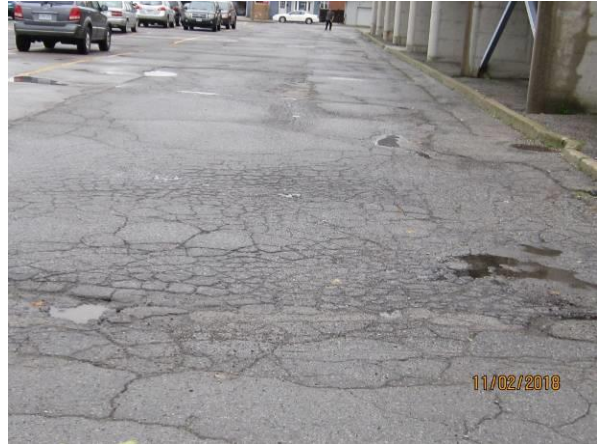
View showing damaged asphalt pavement surface at the north parking lot.
