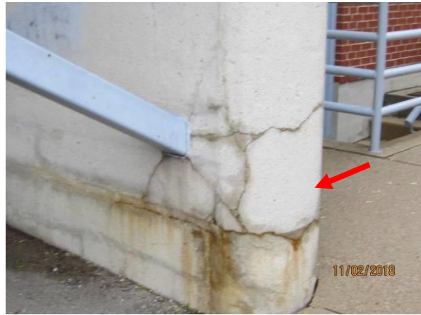
View showing cracked shear walls at the south elevation.
