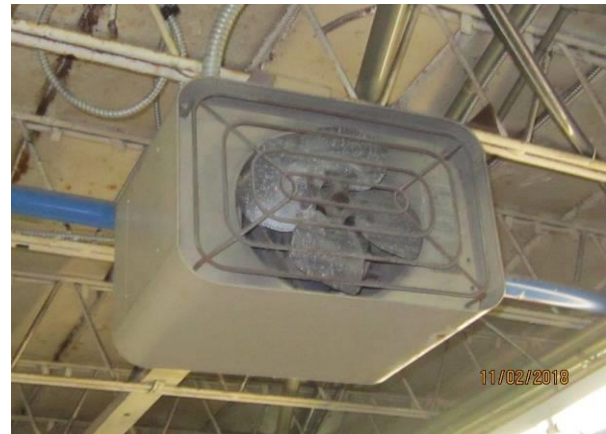
View showing the condition of the ceiling mounted heater in the refrigerator room.
