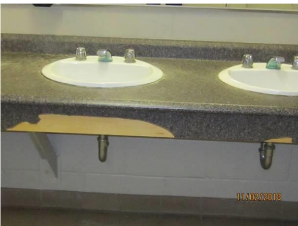
View showing damaged countertop in the women's washroom.
