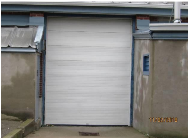
View showing the condition of the overhead door at the west elevation.
