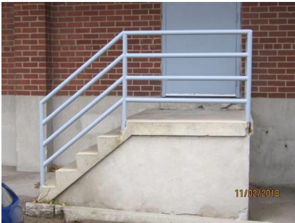
View showing the condition of the metal handrails on the exterior stairs.
