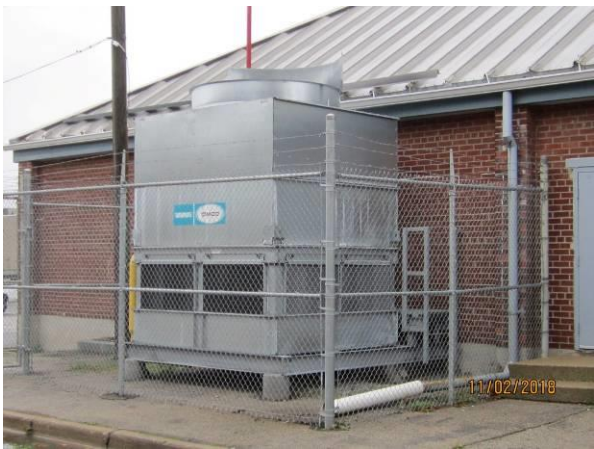
View showing the condition of the chiller unit west of the building.
