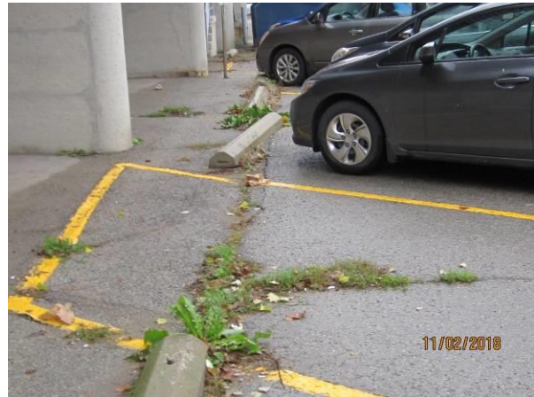
View showing the condition of the precast concrete wheel stops at the south side of the building.
