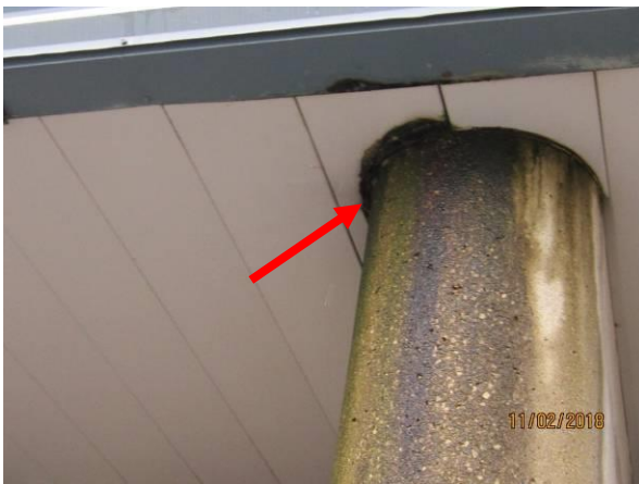
View showing the condition of the metal soffit and draining water around the concrete column.
