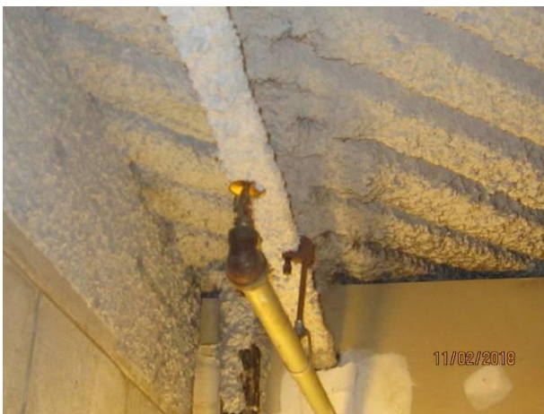
View showing the condition of the metal deck at the office building.
