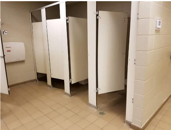
View showing the condition of the partition walls in the washroom area.
