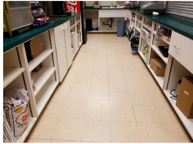
View showing overall condition of the vinyl flooring in Concession Room.
