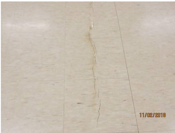
View showing cracked vinyl floor in the hallway second floor.
