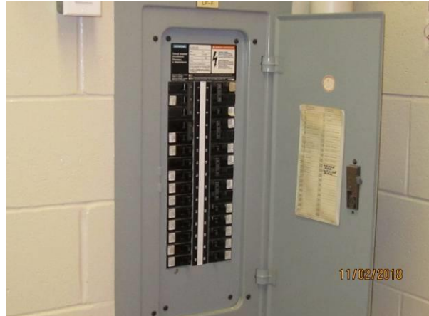
View showing the typical condition of the breaker panels.
