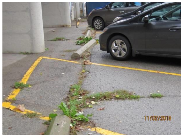
View showing vegetation growth in the asphalt pavement.
