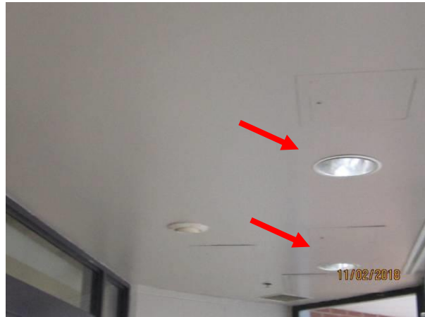
View showing the condition of the interior recessed light fixtures.
