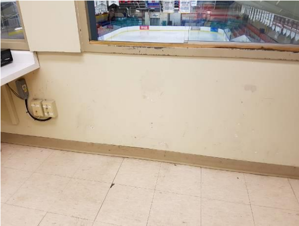
View showing the condition of the drywall in the third floor.
